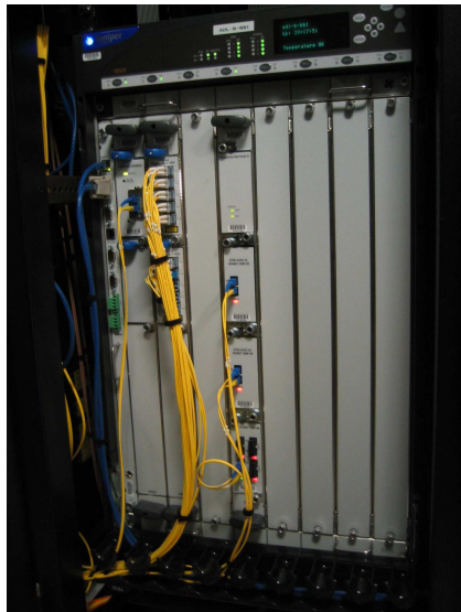
A Juniper router in use.
